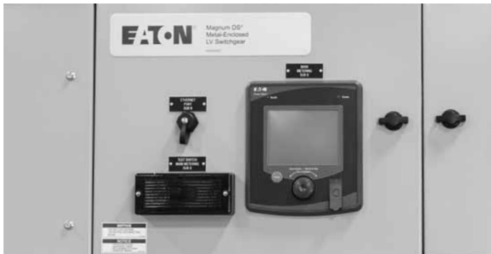
Devices mounted on instrument compartment door
